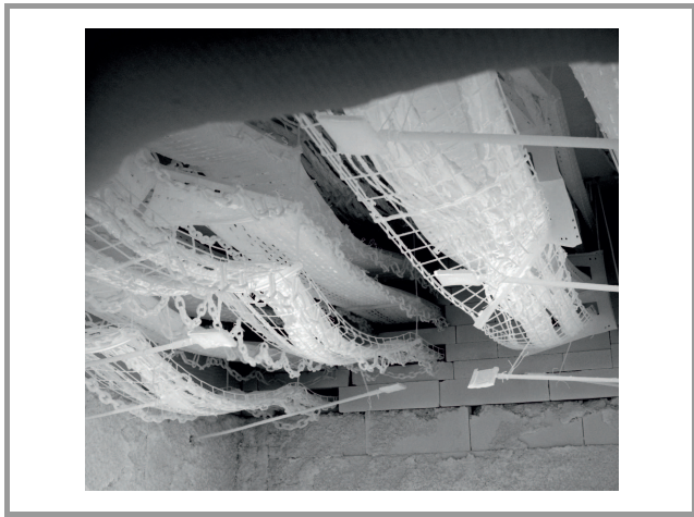
Fig. 4. Interior of a test chamber 25 min after commencing the DIN 4102-12 test. Temperature equals approximately 820°C. The sagging of cable trays is already considerable. The photograph was taken at the FIRES test lab in Batizovce, Slovakia, in 2019. Photo courtesy of Krzysztof Borzycki.
