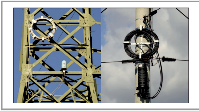
Fig. 8. Spare lengths of aerial fiber optic cable accompanying a joint closure box: OPGW on a 400 kV high voltage power line (left) and ADSS on a low voltage line (right).
